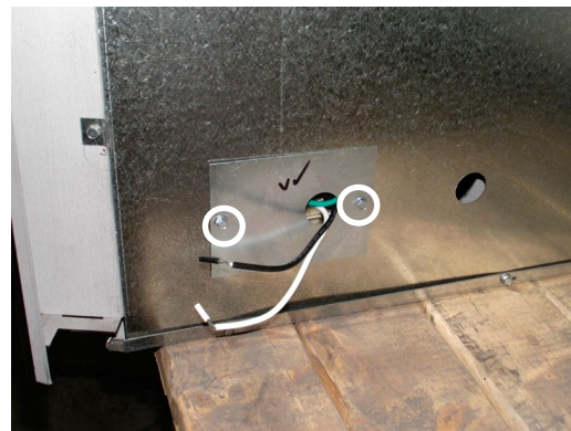
Figure 7 Lead wires that connect to household electrical supply.
